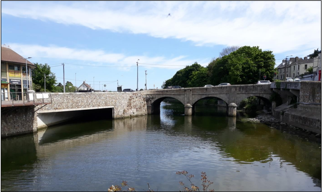
Figure 13 - 3 Arch Road Bridge and Rectangular Culvert at Section 2 and Section 3 Looking Downstream
